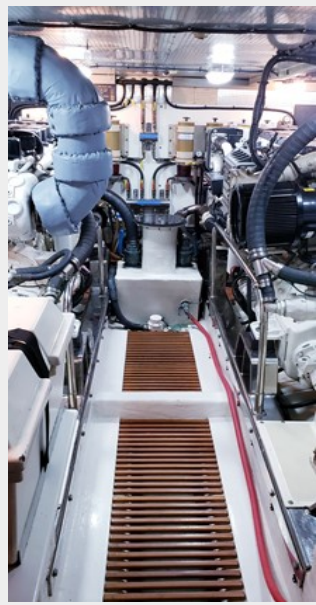
Engine Room Looking Forward
