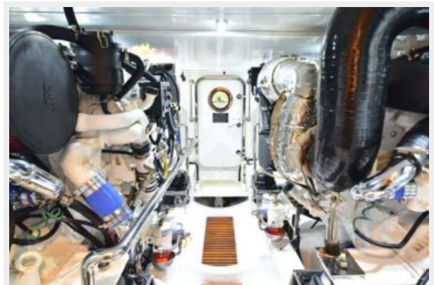
Engine Room facing Forward
