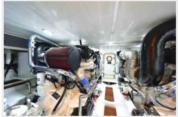
Engine Room Portside
