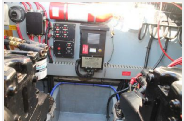
Engine room looking forward
