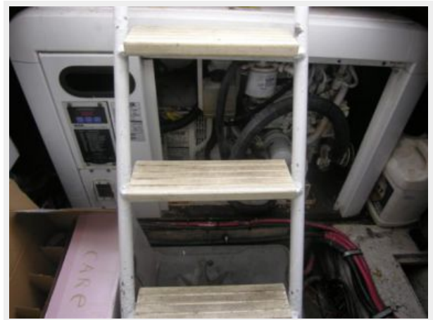
Generator Engine Room
