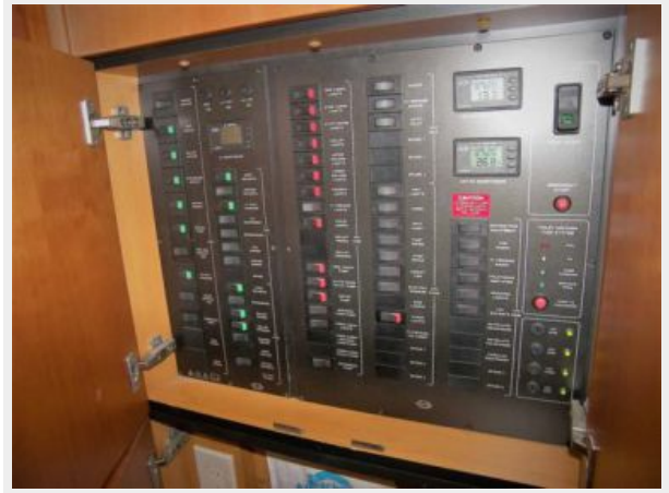
Main Electrical Panel
