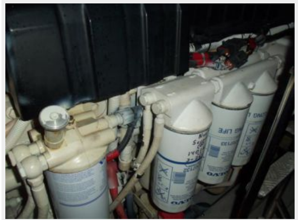
Port Engine Filters
