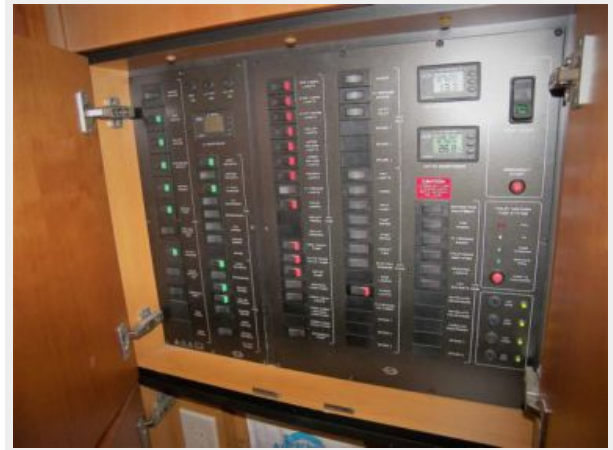
Main Electrical Panel
