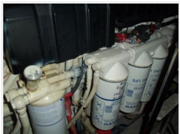
Port Engine Filters
