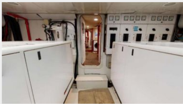
Engine Room Looking Forward
