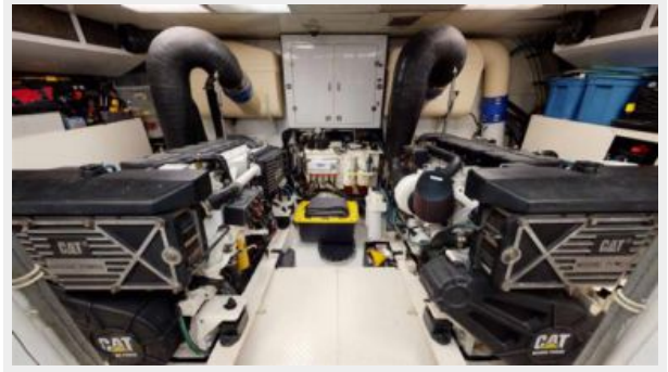
Engine Room Looking Aft
