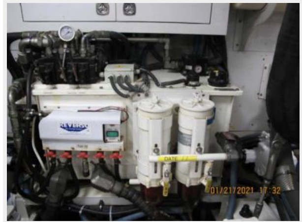
Hydraulic and Fuel Polishing System
