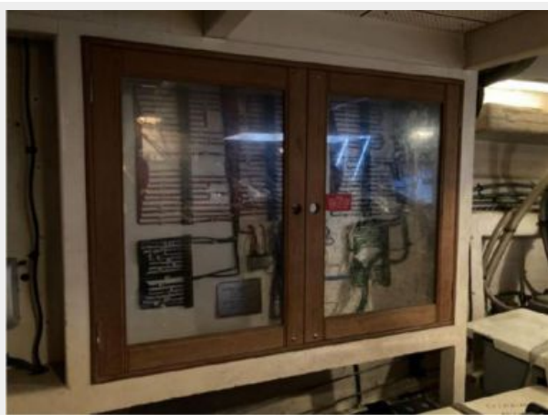
Engine room wiring (2019)
