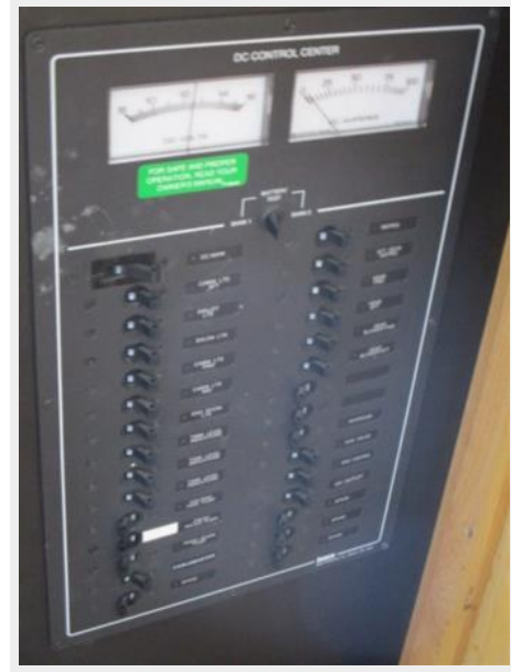
50. Carver 500 DC Control Center
