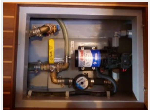
Deck washdown pump with fresh/salt water valve
