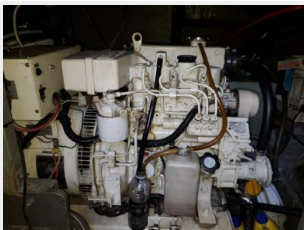
8kW Northern Lights generator
