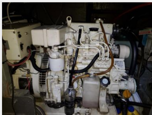
8kW Northern Lights generator
