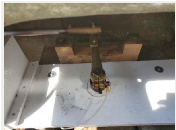
New rudder bearing and support table (port)
