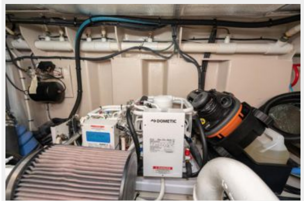
Engine room view 3
