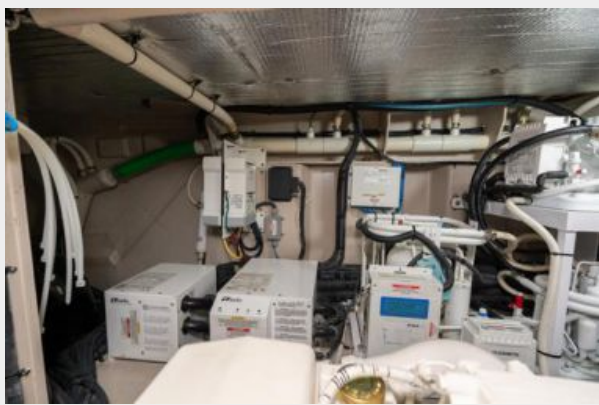
Engine room view 2
