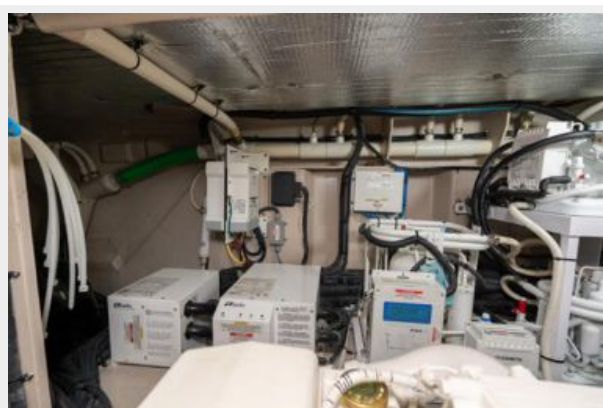
Engine room view 2
