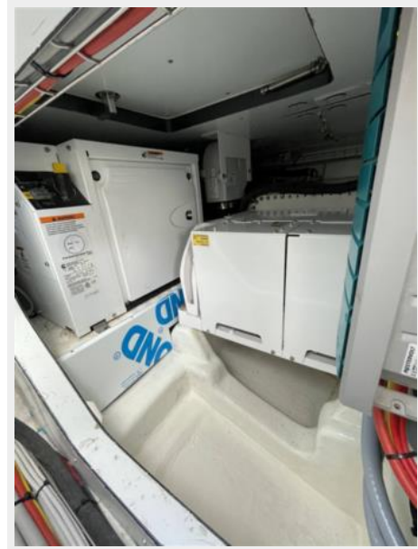
Generator and Gyro
