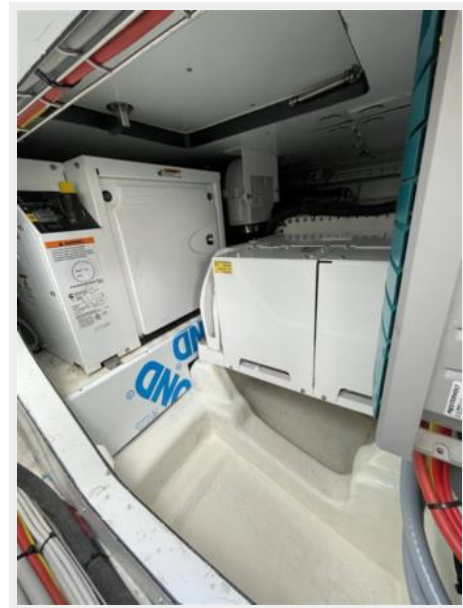
Generator and Gyro
