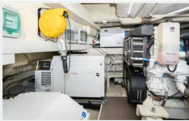
Engine Room - Generator and Watermaker
