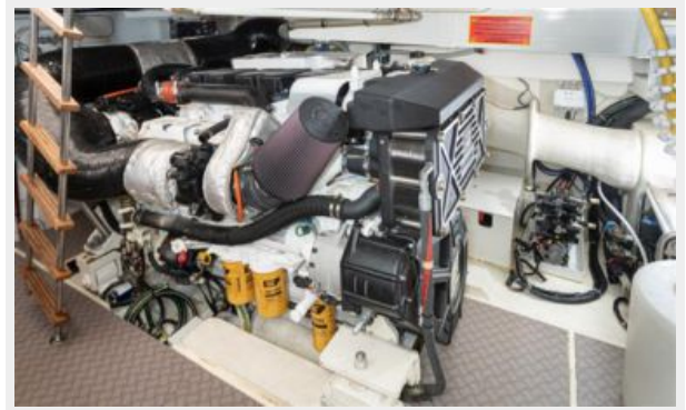
Engine Room - Starboard Engine
