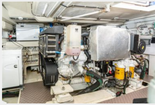
Engine Room - Port Engine
