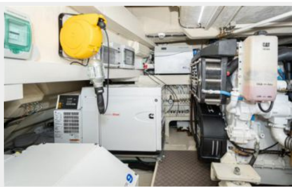
Engine Room - Generator and Watermaker
