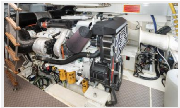
Engine Room - Starboard Engine
