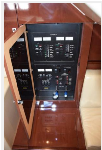
Main electrical panel
