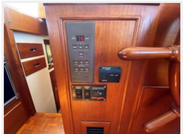
AC Generator Controls
