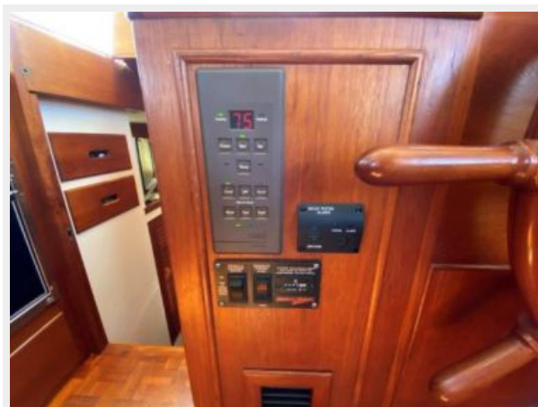
AC Generator Controls
