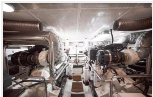
Engine Room Looking Forward
