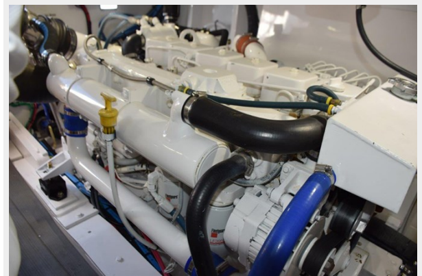
Recent cooling services done
