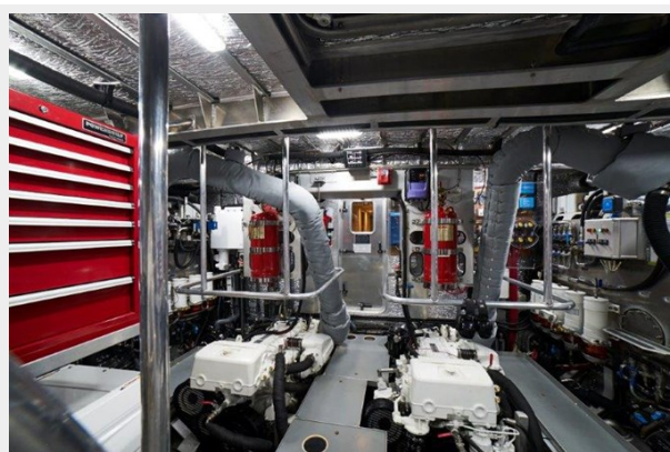
ENGINE ROOM LOOKING FORWARD
