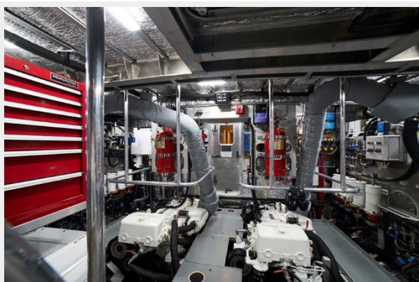
ENGINE ROOM LOOKING FORWARD
