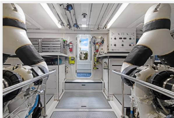
BELLA GIORNATA 94' Lazzara 2000/2018 Flybridge Motor Yacht: Engine Room
