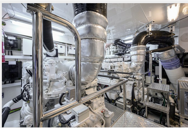
Wiggle Room_Engine Room7
