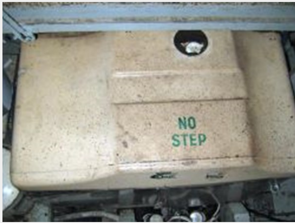
Generator with sound shield
