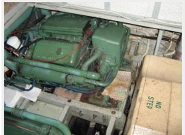
Starboard main engine
