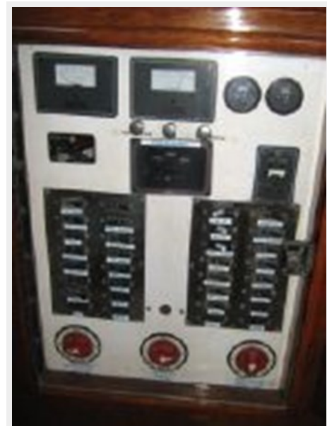
Master electrical panel
