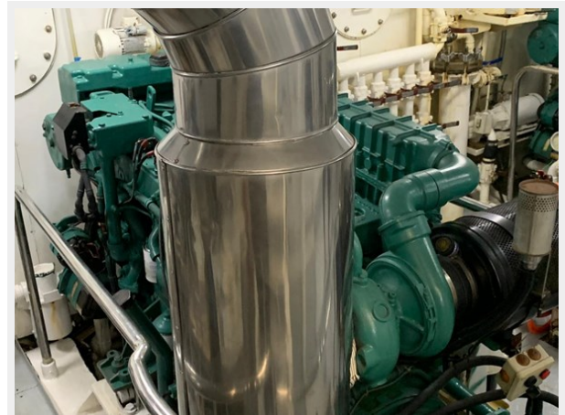
20.Victoria A_engine room5
