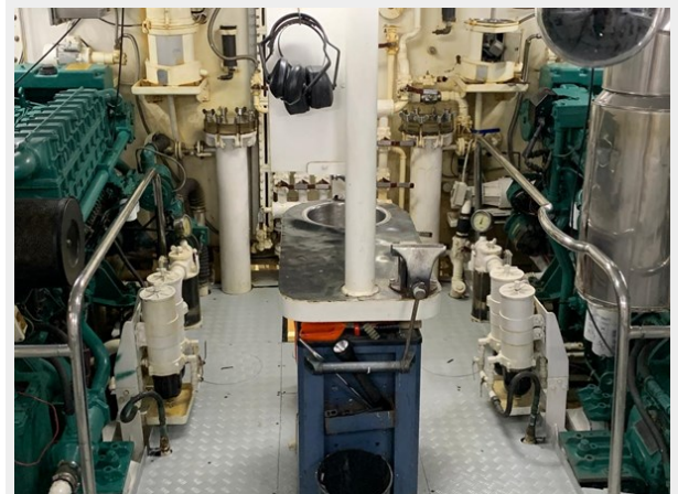
20.Victoria A_engine room1
