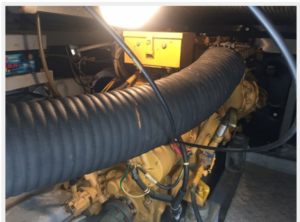
Azimut 36 Fly - Motor Yacht - interior - Engines Room - IMG_1697
