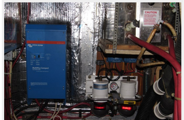
Inverter & fuel filters
