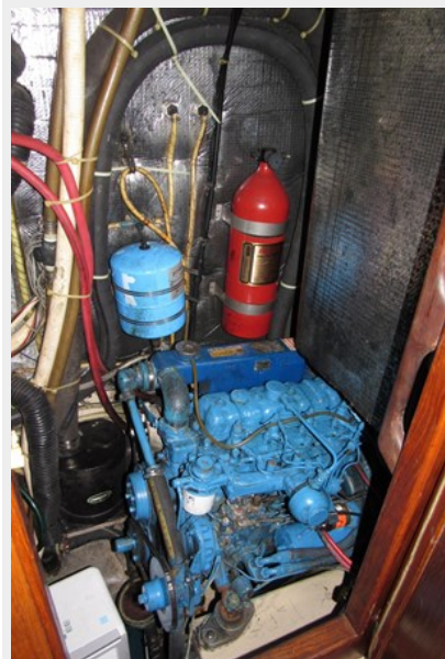
Engine room from walkthrough
