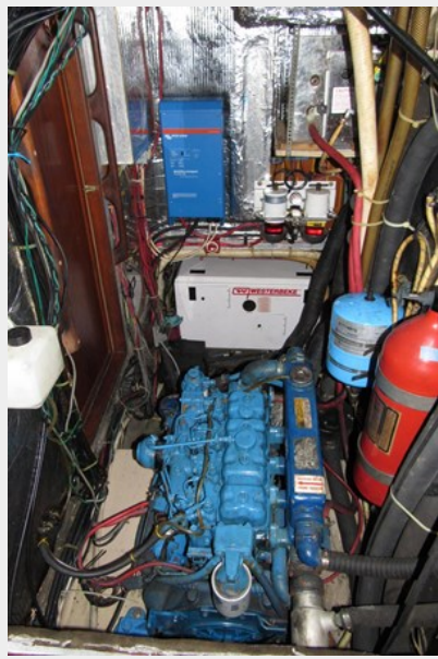
Engine room access from aft cabin
