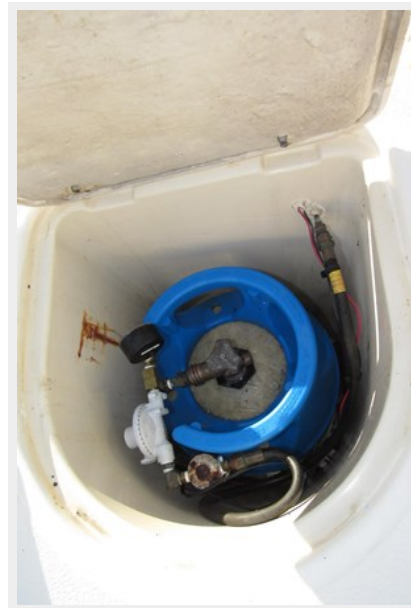
Propane locker (1 of 2)
