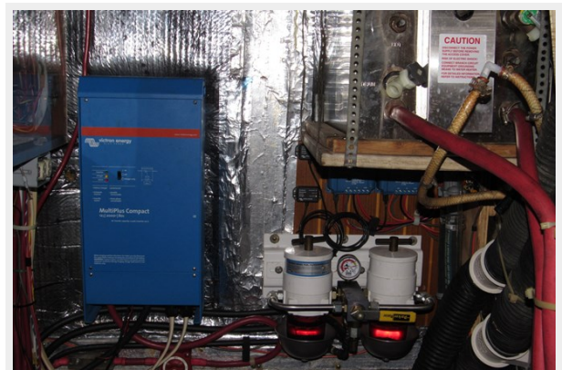
Inverter & fuel filters
