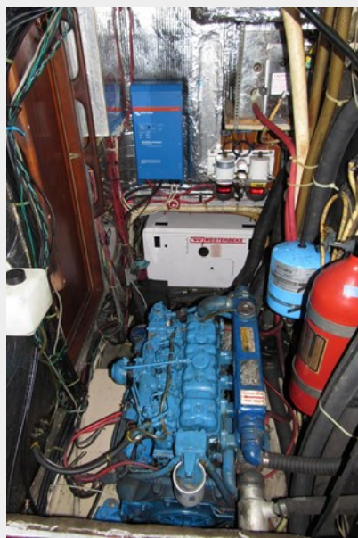
Engine room access from aft cabin
