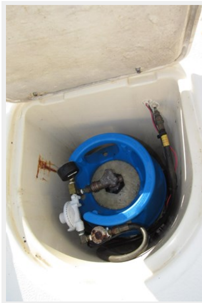
Propane locker (1 of 2)
