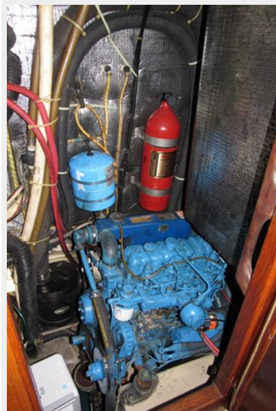
Engine room from walkthrough
