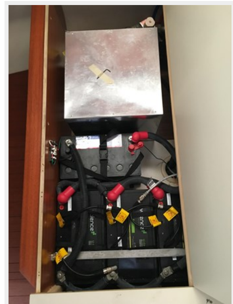
Batteries and water heater
