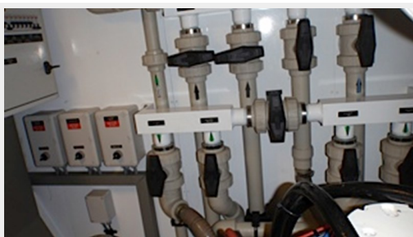
Royal van Dam NORDIA 70 Blue Eagle Engine room V
