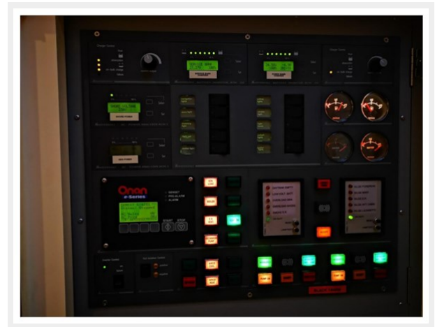
Royal van Dam NORDIA 70 Blue Eagle central system cabinet
