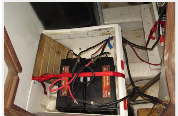
Batteries in Storage under stairs
