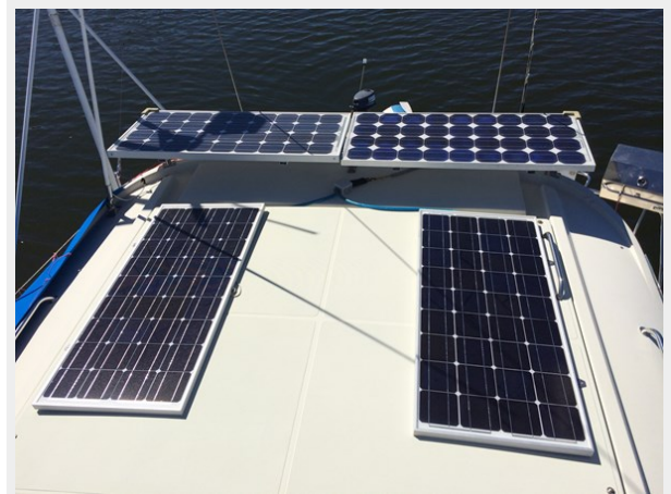
Solar panel array
