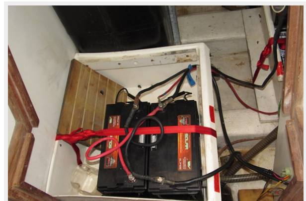
Batteries in Storage under stairs
