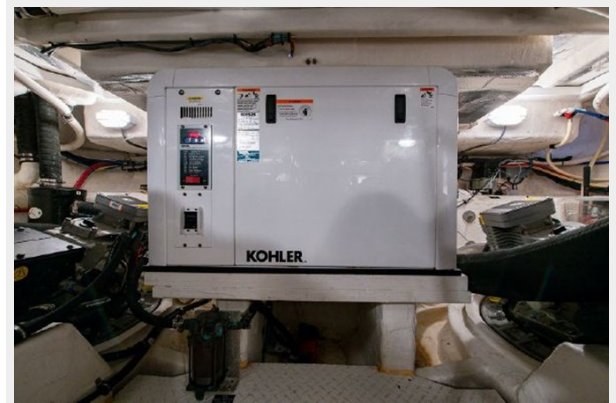
15_Engine Room 4, Generator
