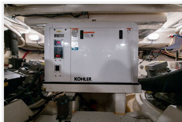
15_Engine Room 4, Generator
