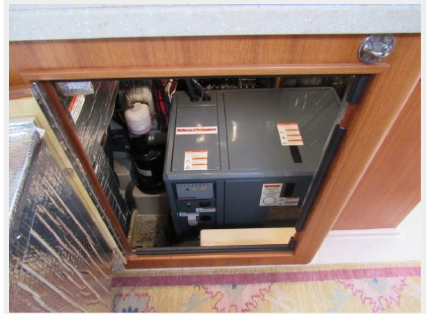
Engine & Generator Access
