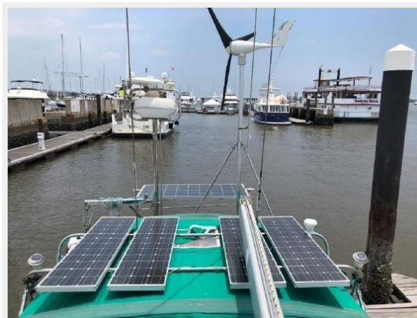
Solar panels and wind generator
