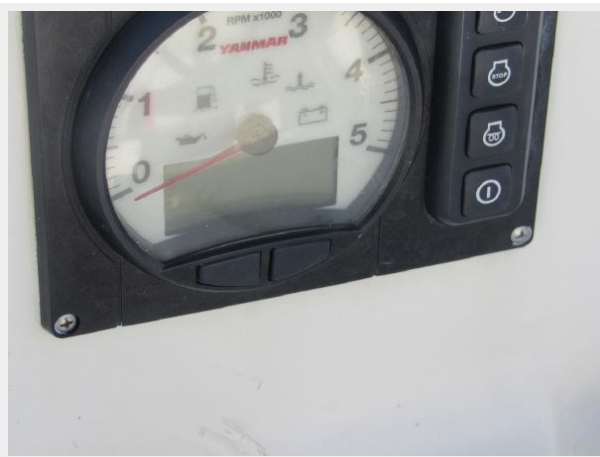
Yanmar Electric Panel
