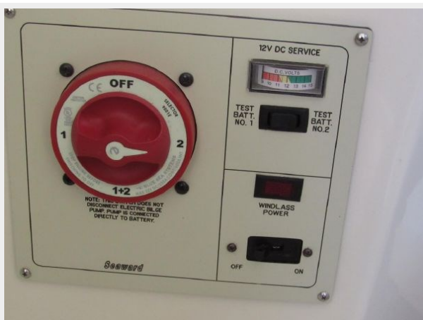
Battery Switch Selector
