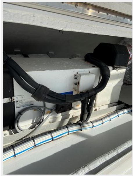
AC in bridge
