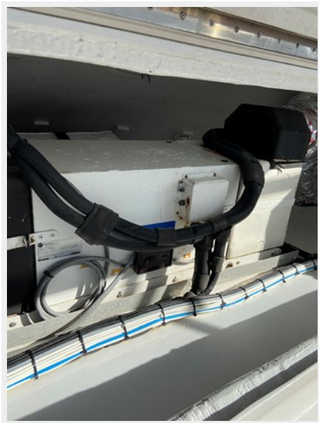
AC in bridge
