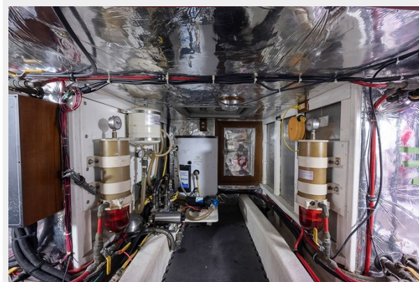
We're Comin'_Engine Room8
