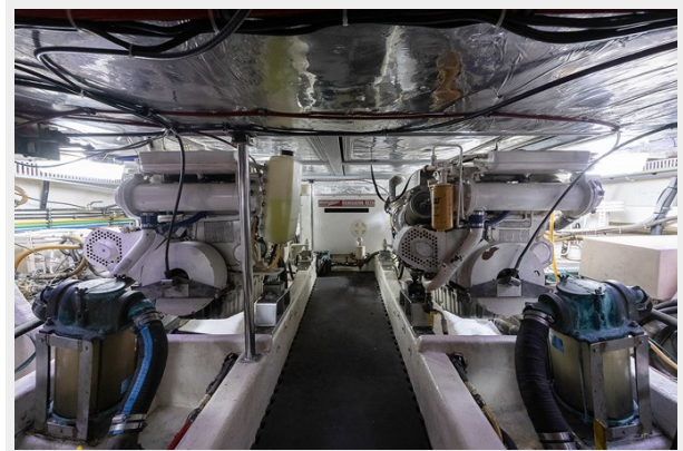
We're Comin'_Engine Room1
