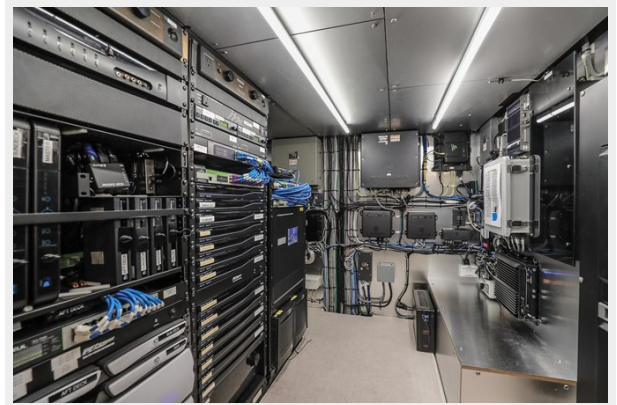
A/V and Electronics Room
