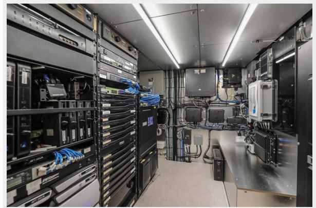
A/V and Electronics Room
