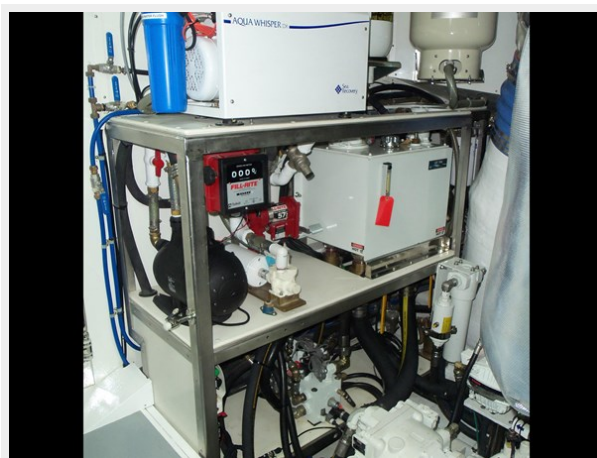
Portside aft equipment
