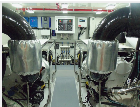
Engine room looking forward
