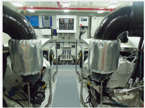
Engine room looking forward
