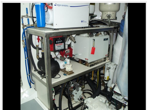
Portside aft equipment
