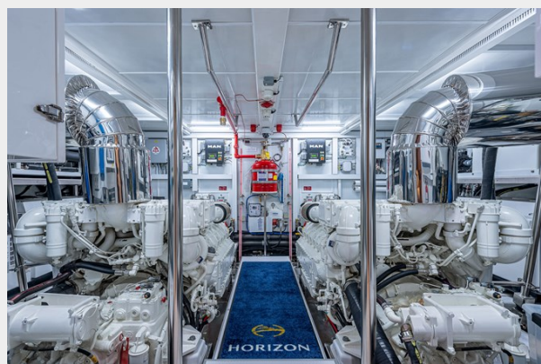
27-E90 Hull 22_Engine Room
